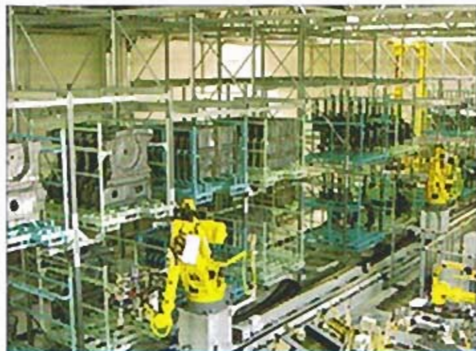
Hochregallager im Body Shop High-shelf warehouse in the body shop
