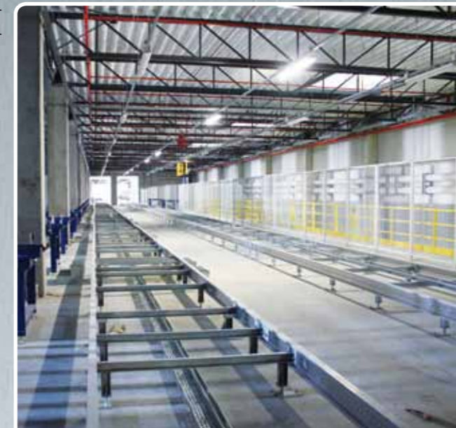
EPB-Strecke zum Hochregallager PPC line to high-bay warehouse
