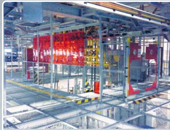
EHB-Hubstation EMS elevator
